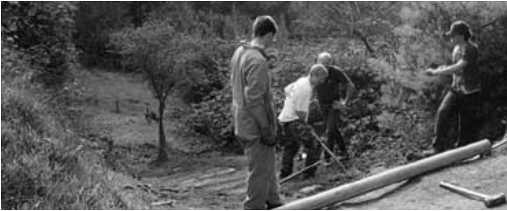
Left: Warren Howe, Maurice Delmar and Ryan Taylor, lead by Paul Maheu of Troop 19 grade and lay wooden steps to the steep slope of Keelar Avenue Path.
