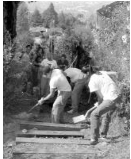
University of California, Berkeley students install steps on Atlas Path as part of Cal Corps, October 20th public-service day.
