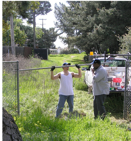
Parks Dept workers open fence on the Santa Fe Right of Way at Lincoln St.
