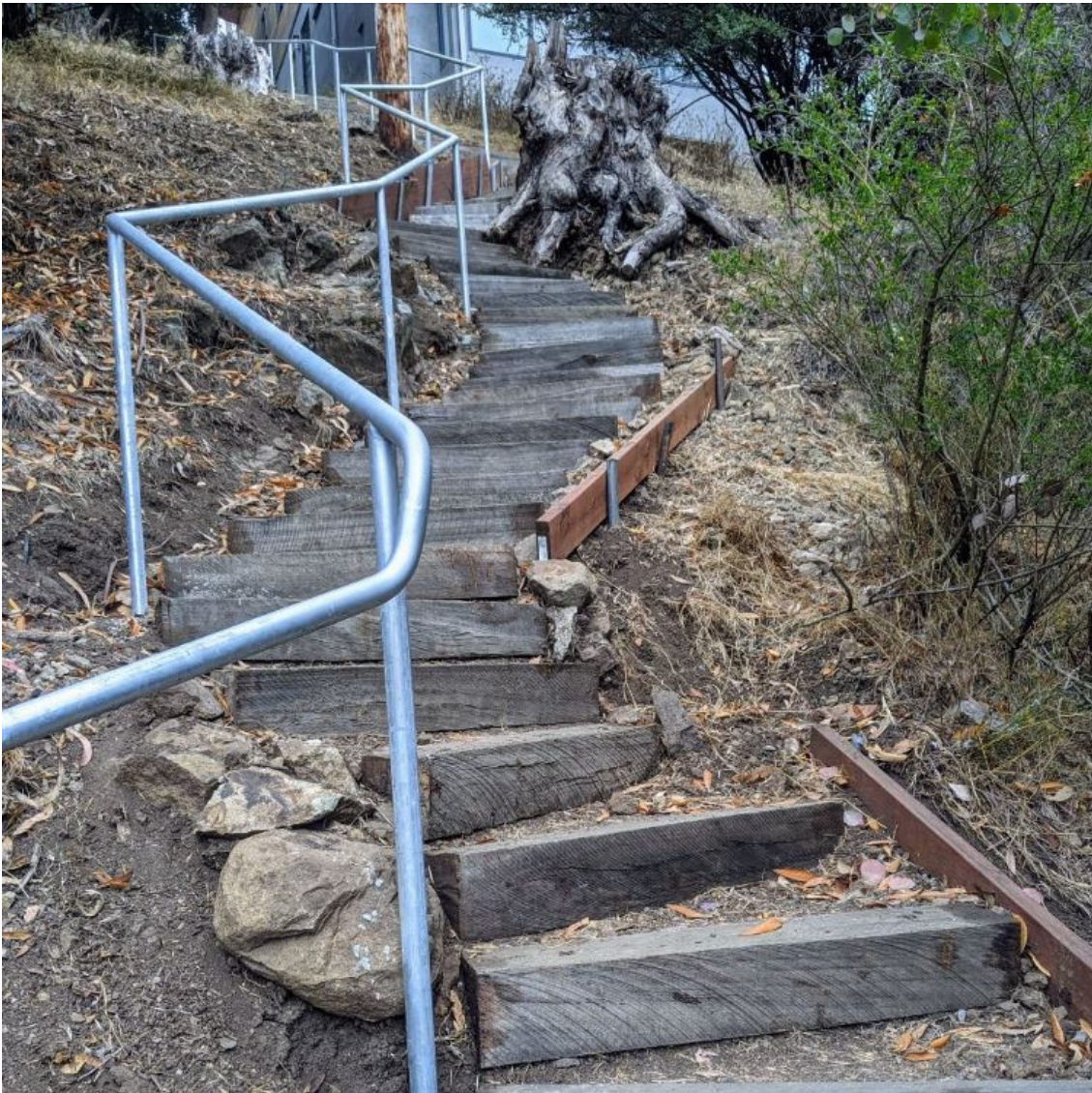
Above, the new handrail installed by Berkeley Path Wanderers Association on Columbia Path.
